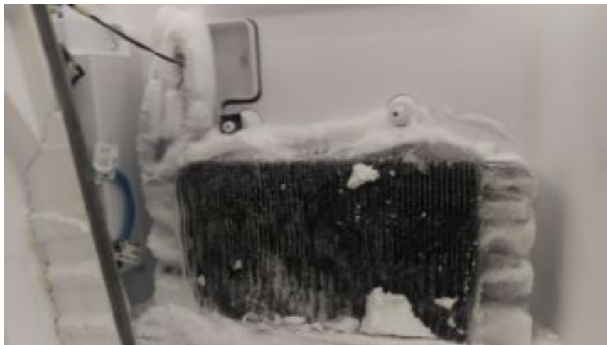
Figure 3 - FROSTED REFRIGERATOR EVAPORATOR AFTER COVER REMOVAL
