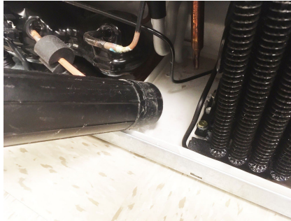
Figure 4 - DRAIN PAN WATER REMOVAL
